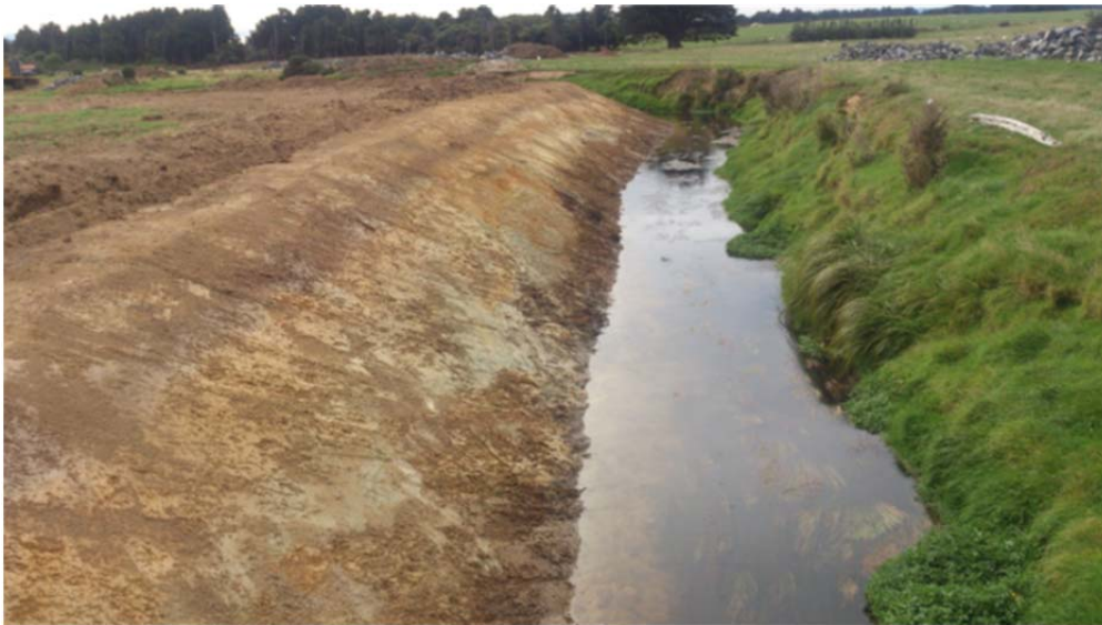
Figure 17. Example of the bank reconstruction (re-battering) works in progress in Waituna Creek (photograph taken from the middle of Site 3F looking upstream).
