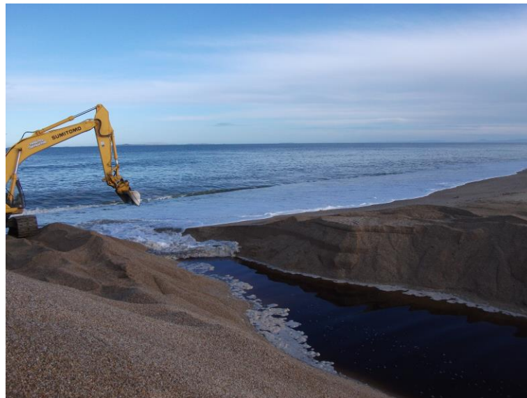
Figure 1 A digger opens a cut in the Waituna Lagoon sand bar, 2013 (photos: K. Robertson).
